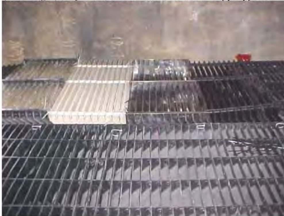
Figure 2. Test Installation at APS's Cholla Station, Unit 2: Materials (left to right) Polysulfone, FRP, Stainless Steel, Polypropylene
